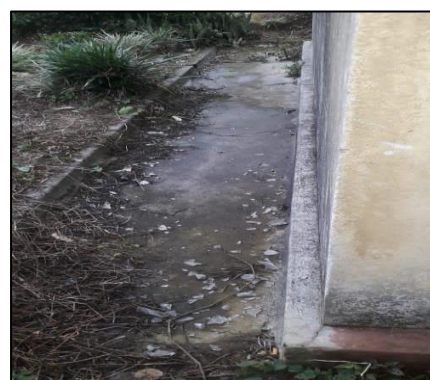
Figure 10: Improper maintenance of drainage
